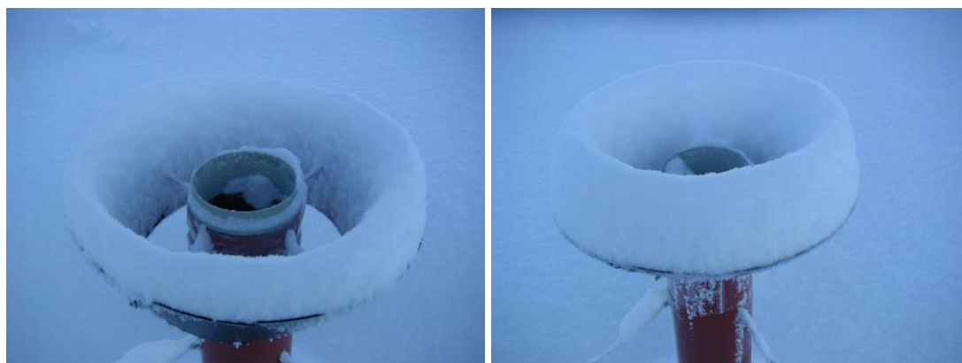
Figure 19. Snow on the wind shield of the bulk collectors.
